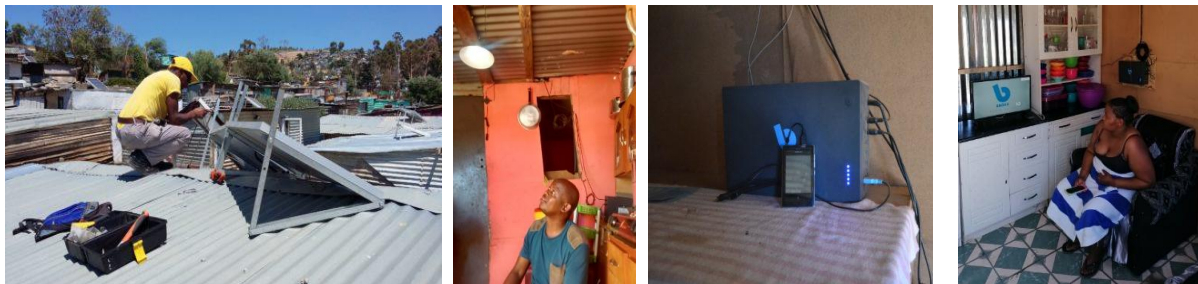
Figure 13: Photos of iShack off-grid solar home system installations
